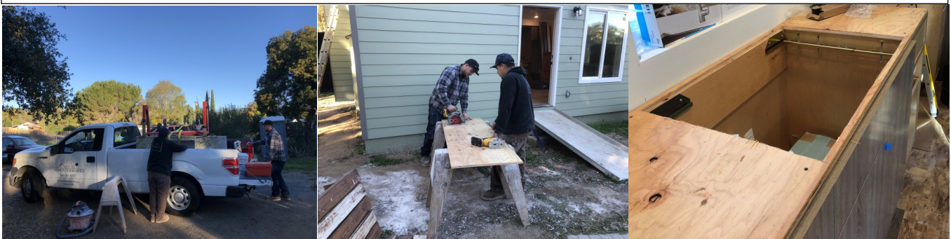
On November 29, Jesse's colleagues, Dylan and Jaime, arrived to install the countertop. The first step was cutting a hole in the plywood subtop for the installation of the undermount sink.
