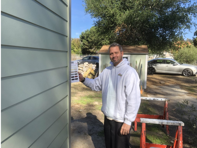
Chris Krajewski, Manager of Rain Gutters for Santa Fe Roofing & Rainutters , came to the site on October 21 to take measurements for our rain cutters and did a color match with the fascia and trim on our cottage.
