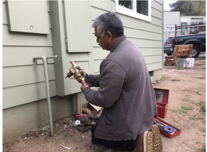
On November 5 Flo Echeverria, Service Technician for Symons Fire Protection , came to the site to install a pressure regulator for our fire protection system, because our water pressure can exceed 150 psi.
