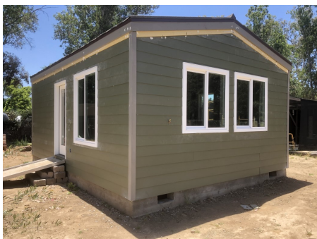
Our Wounded Warrior Homes Cottage under construction: a 400 sf permanent structure Tiny House.
